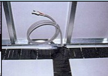
2. Extrusion from Cable Trenches to dry wall or demountable partitions.
