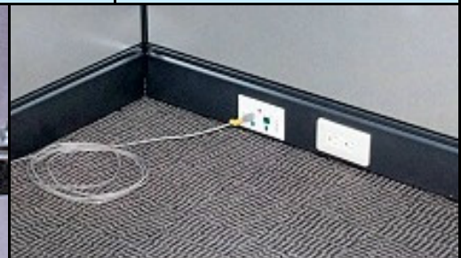
3. Extrusion from Cable Trenches to exit wall base.
